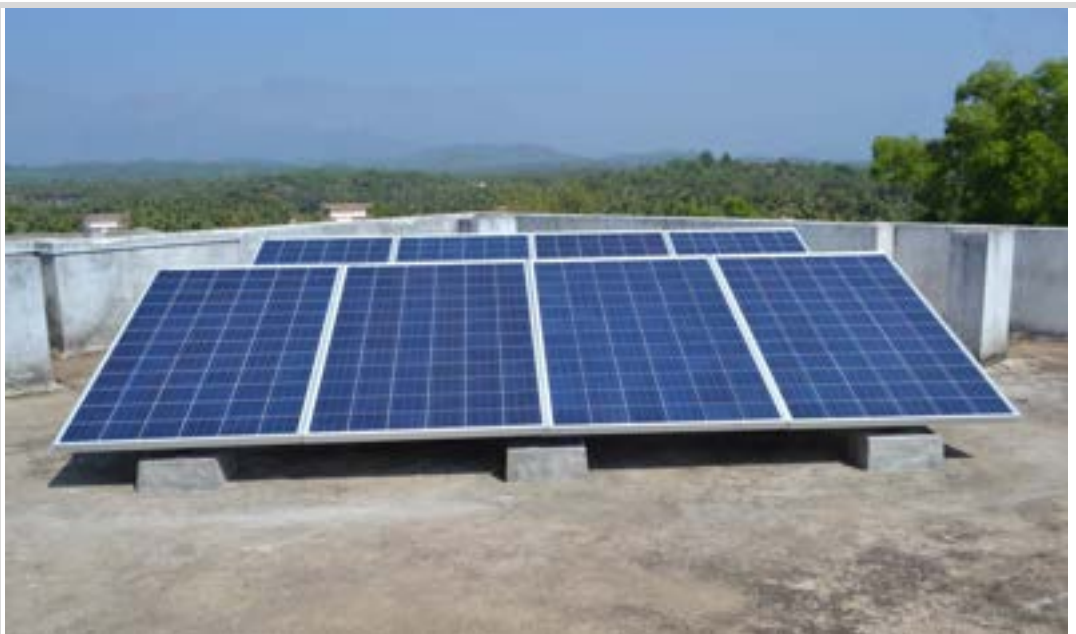
225 kWP ROOF TOP SOLAR PHOTOVOLTAIC POWER PLANT
