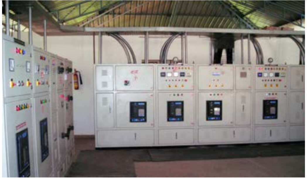
POWER HOUSE CONTROL PANELS 320kVA and 500kVA generators
