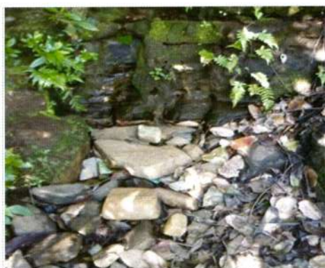
Soil Pipe flow
